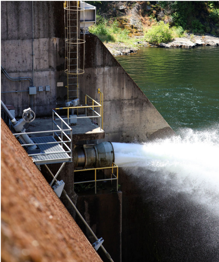
Ralston Afterbay Stream Maintenance Valve
