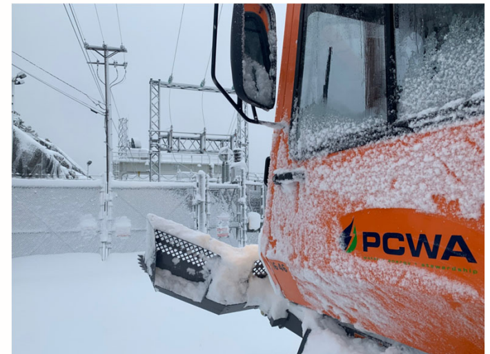
French Meadows Powerhouse
